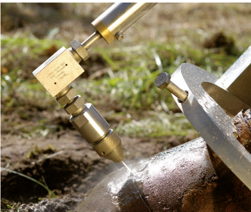
Cutting with Base Fuse Manipulator
